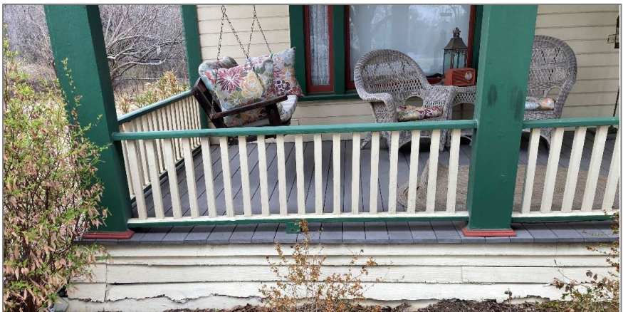
FIGURE 2: APPLICANT'S PHOTO OF CURRENT SKIRT DECAY
